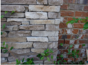
Vertical cracks in stone
