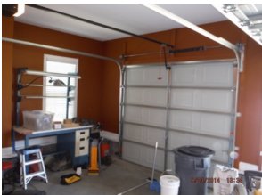
Front garage overhead door
