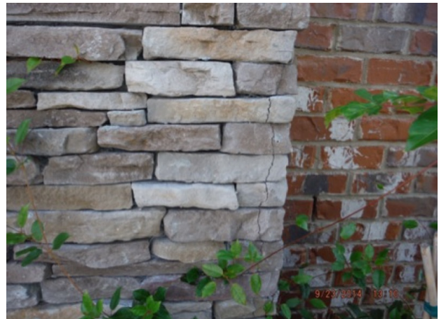
Vertical cracks in stone
