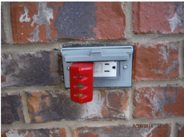
No power at front porch GFCI receptacle
