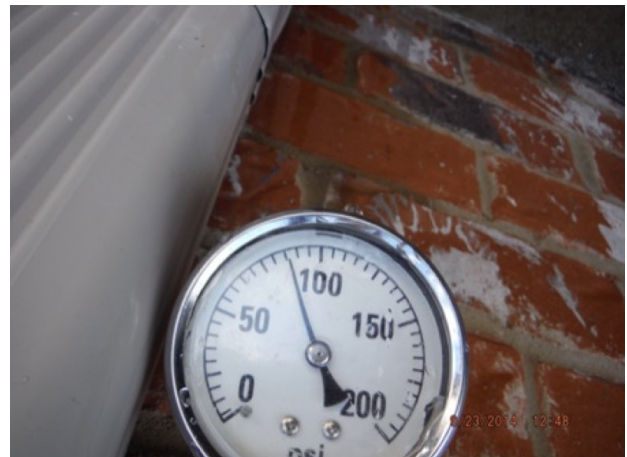
Water pressure is higher than 80 p.s.i.
