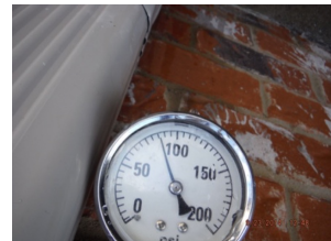
Water pressure is higher than 80 p.s.i.
