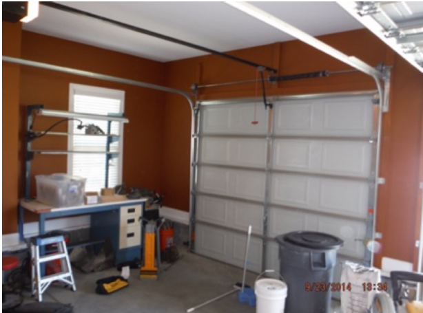
Front garage overhead door
